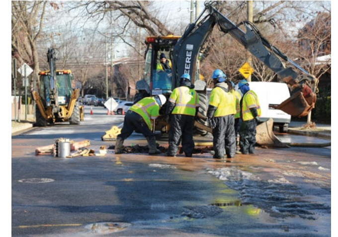
In FY22 we used equity criteria to update our prioritization of the inspection and rehabilitation of small diameter water mains and local sewers over the next 10 years
