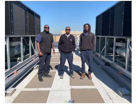
HQO chiller replacement project. L-R: Harold Jusse, New AC Mechanic 10, William Shackelford, New HVAC Foreman, Matthias Frazier, AC Mechanic 10, flanked by two new chillers at the CMF building at Blue Plains.
