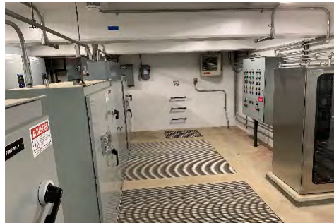
New Electrical & Control Panels at 14 th St. Bridge Pump Station
