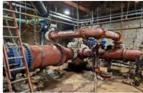
Reclaimed Effluent Pump Station Upgrade
