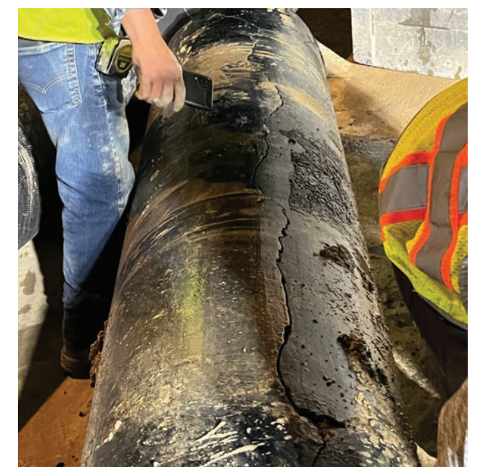
Split in a 115 year old cast iron pipe
