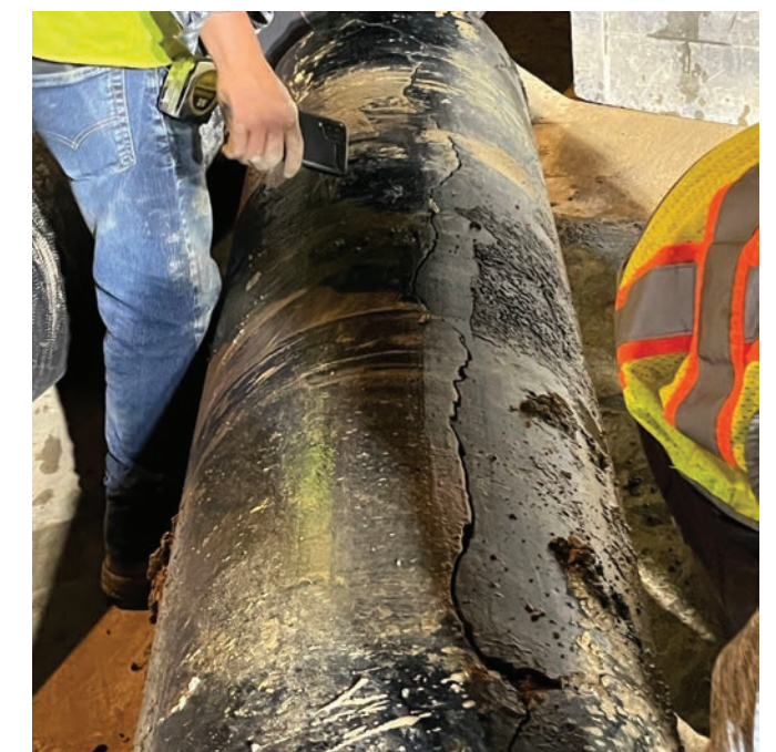
Split in a 115 year old cast iron pipe
