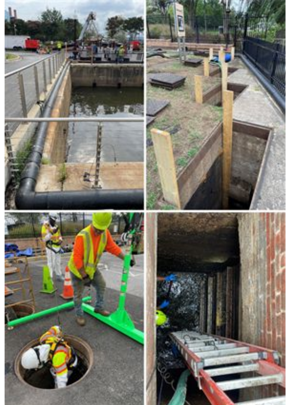
Installation of temporary bypass piping & diesel pumps, metal plate installation to control water levels, channel structural inspection, and Tide Gate structural inspection.
