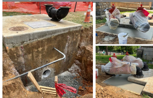
Emergency Booster Pumping – Ft. Reno PS
