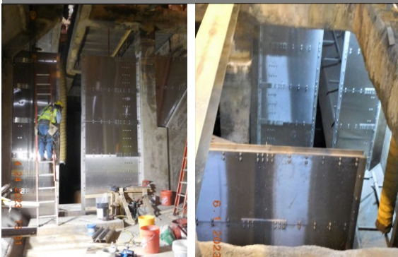
Grit Chamber Baffle Wall Project
