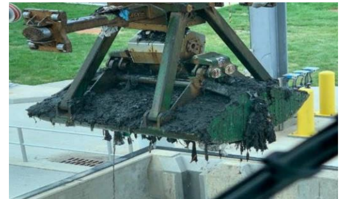
Trash, Debris and Solids Removal from Screening Shaft at Tunnel Dewatering Pumping Station
