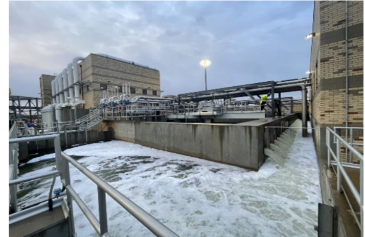
Enhanced Clarification at the Wet Weather Treatment Facility
