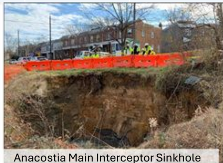
Anacostia Main Interceptor Sinkhole
