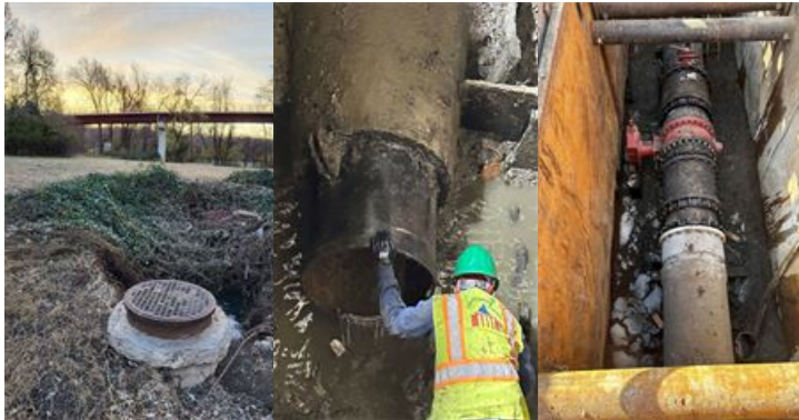
Pipe break on 30" pipe in Anacostia Park
