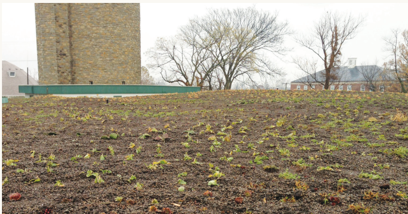
Recently constructed and planted green infrastructure roof at Fort Reno mimics natural processes to control stormwater
