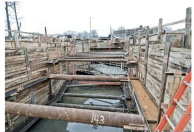
DC WASA CONTRACT 110210 CORMAN CONSTRUCTION, INC. © BERKSTON ASSOCIATES, PHOTOGRAPHERS WASHINGTON, DC DATE: 12/10/12 PHOTO NO. 18-203 DESCRIPTION: LOWER APPROACH CHANNEL AREA
