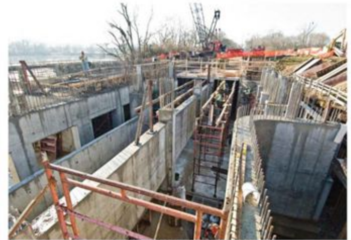
CONTRACT NO. DC WASA 11000 SULLIVAN SCHULTZ CONSTRUCTION LLC 8800 WASHINGTON AVENUE, WASHINGTON, DC DATE: 12/18/13 PHOTO NO. 35-327 DESCRIPTION: OVERFLOW STRUCTURE UPPER DECK SHORING + S
