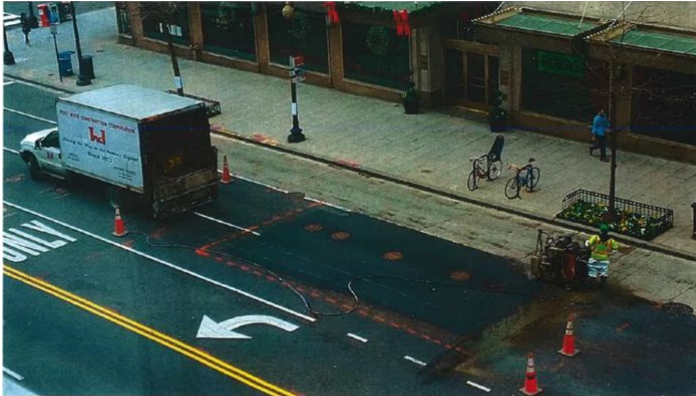
12-11-15 Fort Myer is on-site saw cutting the South Excavation. South side work consisted of installing a new 24" Butterfly Valve, 1-Air blowoff assembly and 1-Drain blowoff assembly. Crew will be removing the temporary asphalt to the marked limits as discussed with DDOT inspector.
