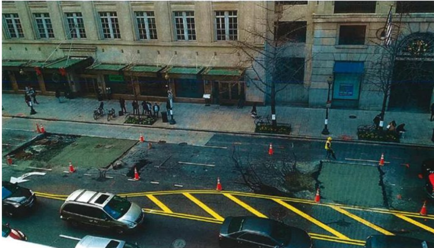
12-11-15 Fort Myers has poured the concrete base around the north excavation and have poured the majority of the South excavation. 2nd concrete truck is needed to pour the remaining concrete pad on the South excavation. First truck arrived on-site at 2:30pm and the last truck arrived at 4:22pm.
