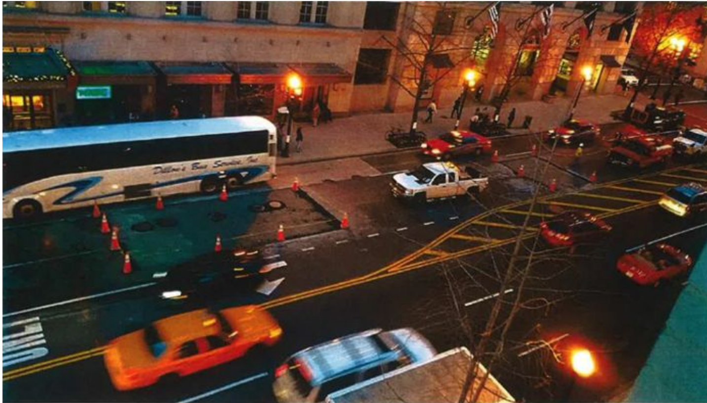
12-11-15 Both the North and South Excavation base pours have been completed. Crews are waiting for the steel roadway plates to cover both excavation. The concrete will be ready for traffic by Monday morning.
