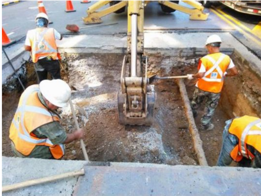
Large Valve Replacements & PRV's Contract 11R - Contract #140070 08/13/2015 - Job Progress Photo # 114 Location 11-6 14th & G St Excavation for Tie-In
