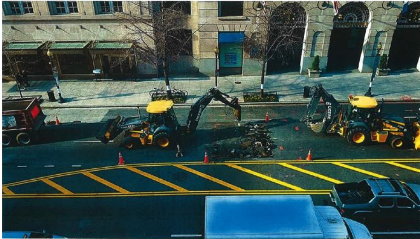
12-11-15 Fort Myers Crew is starting the removal of the temporary asphalt in preparation for the concrete base pour. Above, the Hoeram is removing the temporary asphalt within the saw cut limits. Once complete the Backhoe will load the debris onto the dump truck for site removal.
