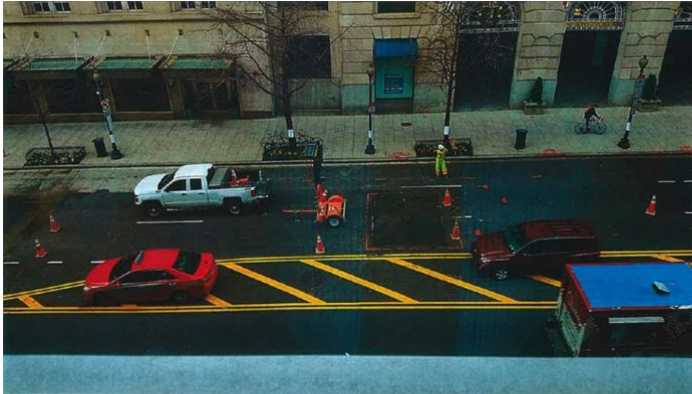
12-11-15 Fort Myers preparing to Saw cut the North excavation per the approved limits discussed with the DDOT inspector. North side work consisted of disassembling and removing the existing 2 EA 24" couplings, 24" Butterfly valve , 2EA 2" air taps and existing manhole. Crew then installed 2EA 24" couplings and a 3' piece of DIP
