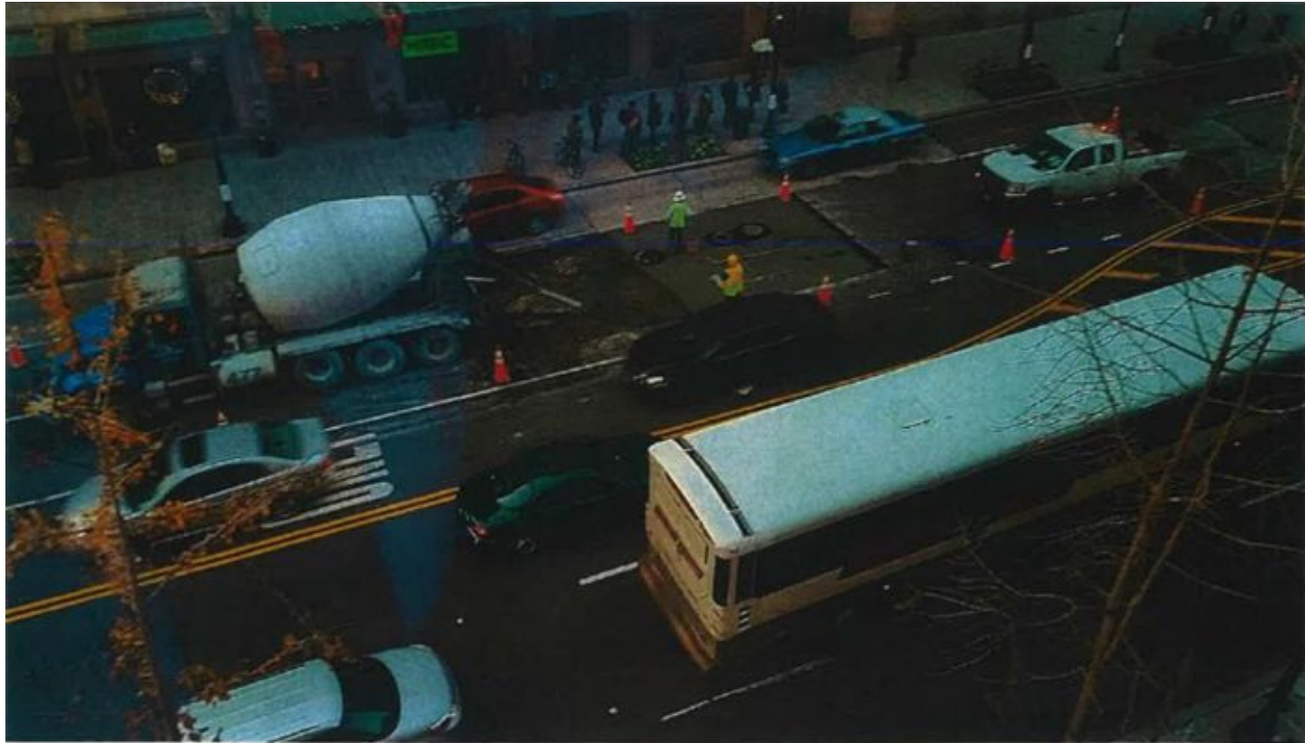
12-11-15 Second concrete truck has arrived at 4:22pm to complete the remaining concrete pour on the South excavation.
