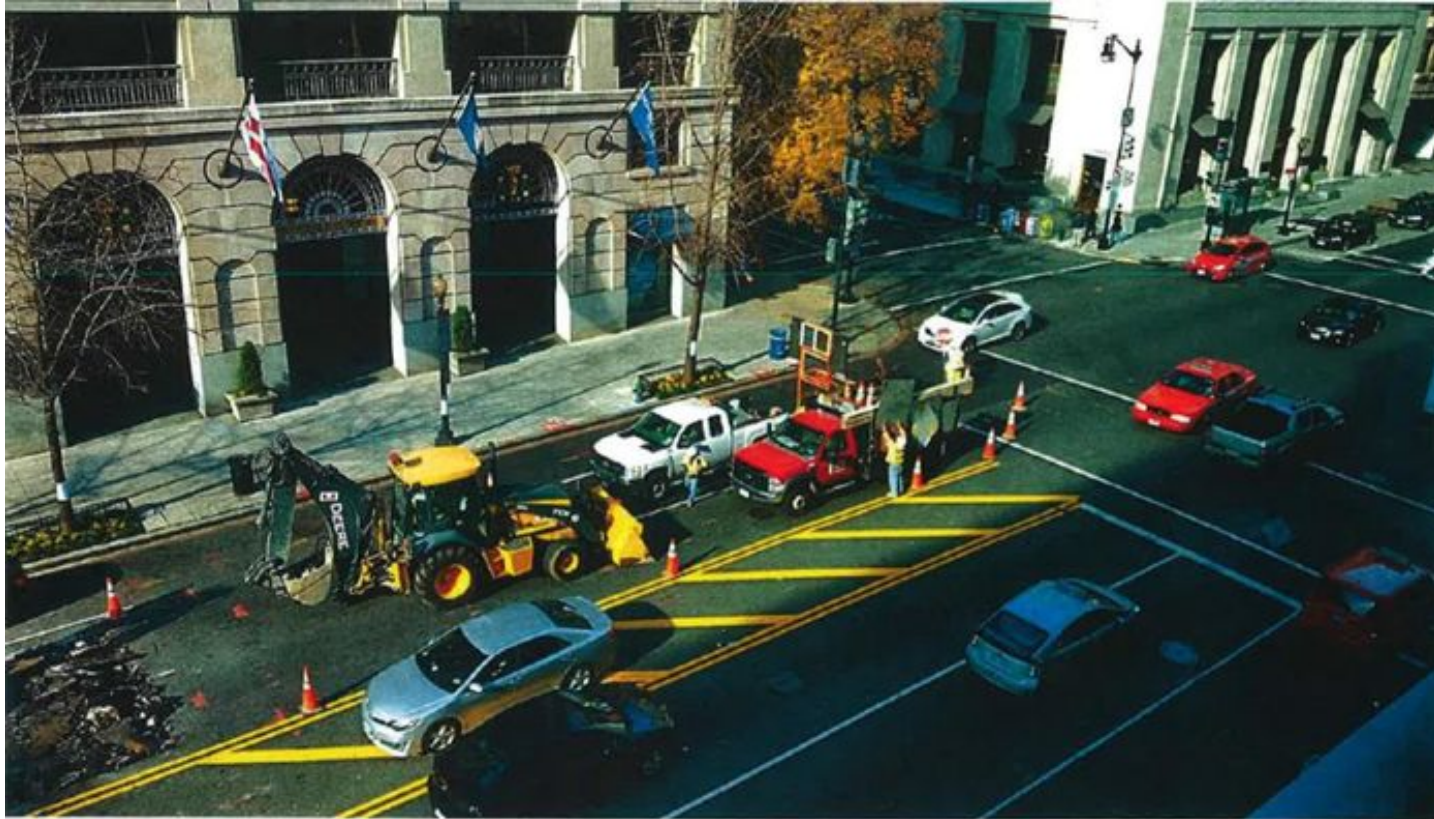
12-11-15 Fort Myer is removing the temporary asphalt debris from the South excavation in preparation for the concrete base pour (pcc). Crew will compact the base soil and place the required wire mesh and dowels prior to the concrete pour.
