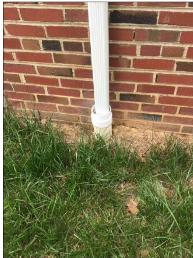
Downspout Connected to Combined Sewer System
