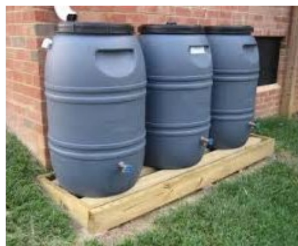
Downspout Disconnection and Rain Barrels
