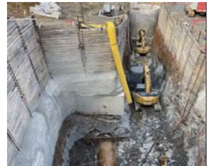
Overview of the open excavation from the new MH30.59 looking down to the new MH31
