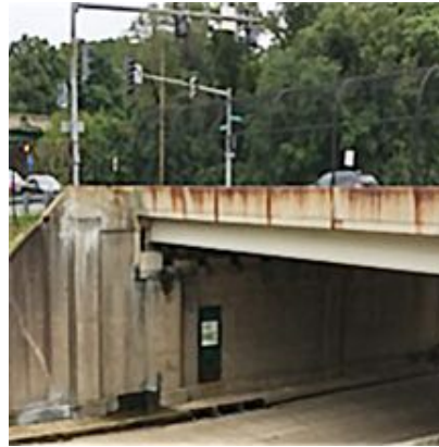
Portland Street Pump Station at South Capital Street underpass at Malcolm X Ave, SE.
