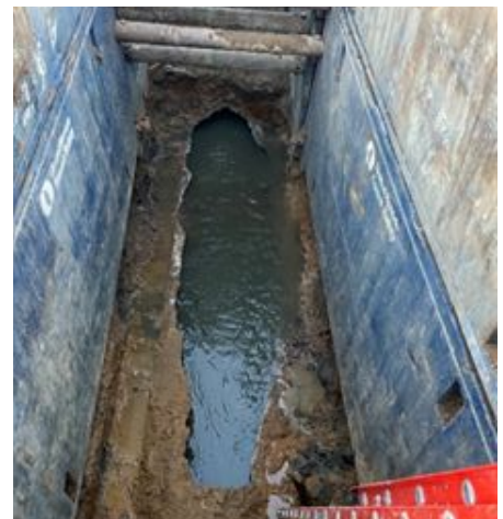
Figure 2: Collapsed Pipe After Site is Secured
