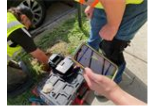
43 properties participated in LFDC's pipe material testing pilot.
