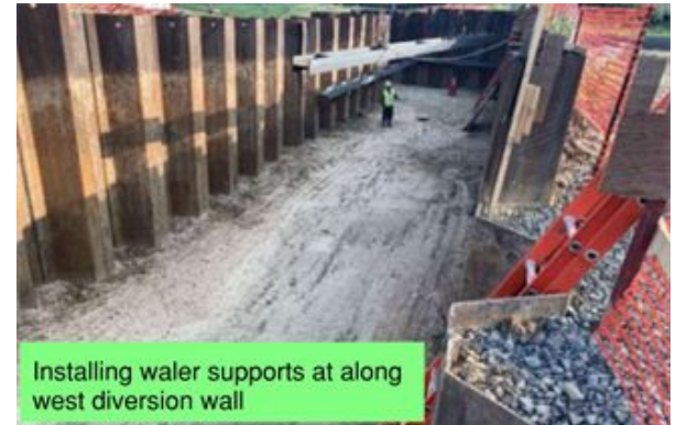
Anacostia Main Interceptor
