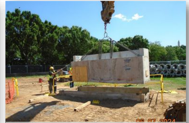
Storm Drain Structures for Bypass Road
