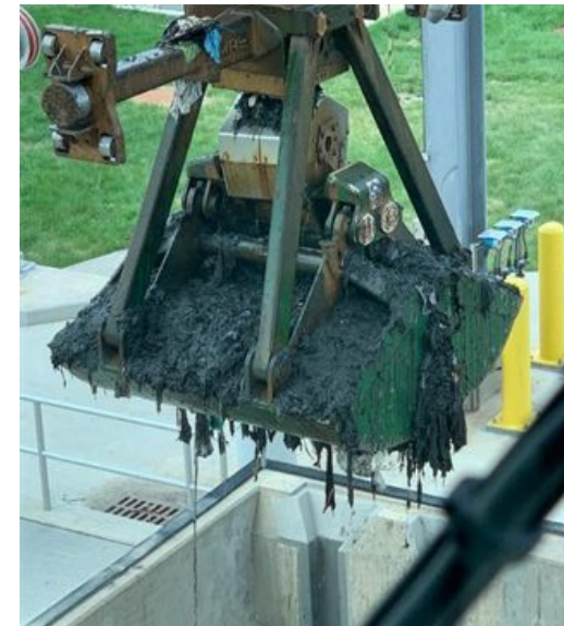
Trash, Debris and Solids Removal from Screening Shaft at Tunnel Dewatering Pumping Station
