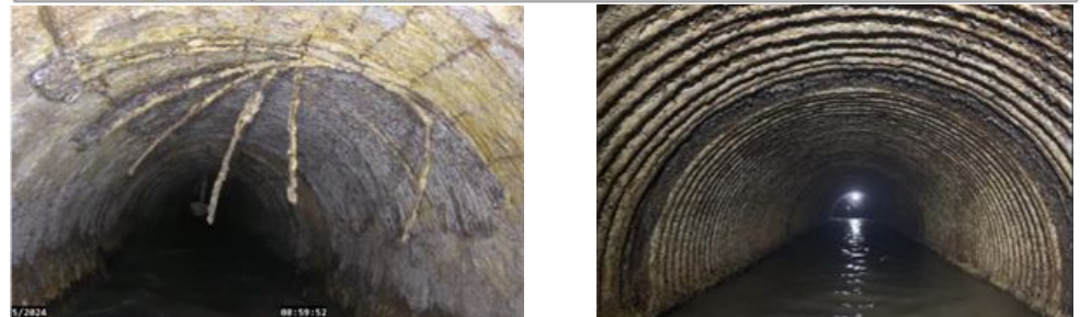
Potomac Interceptor Corrosion Resulting in Loss and Exposure of Reinforcing
