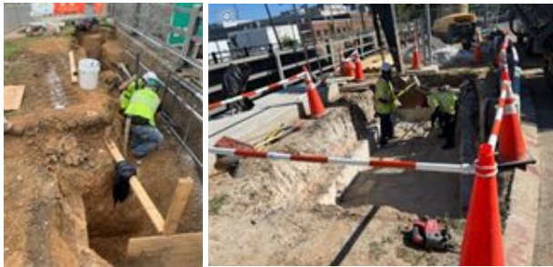
Excavation and installation of rebar for concrete slabs for DC Water I&C and PEPCO cabinets.
