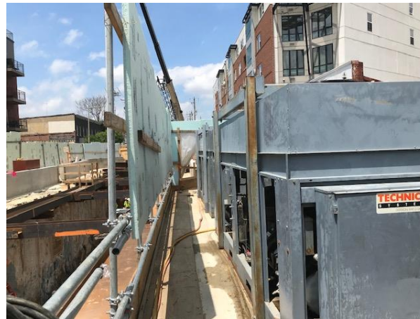
Soil freeze system behind noise barriers
